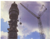
In view of 70 billion Telecom's investment in a digital phone system, it's not surprising that a dish is needed to position high up on the Telecom Tower.
